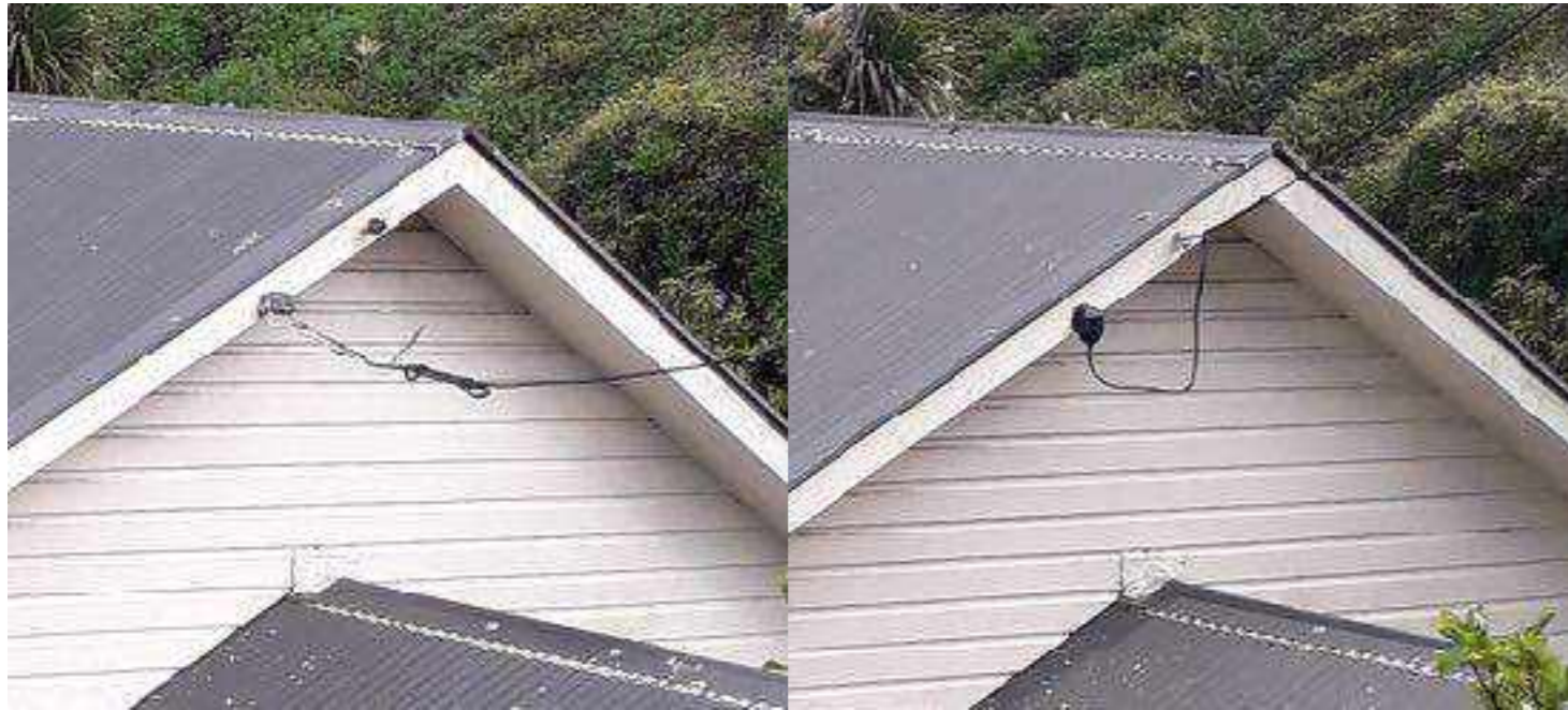
Power supply cable
